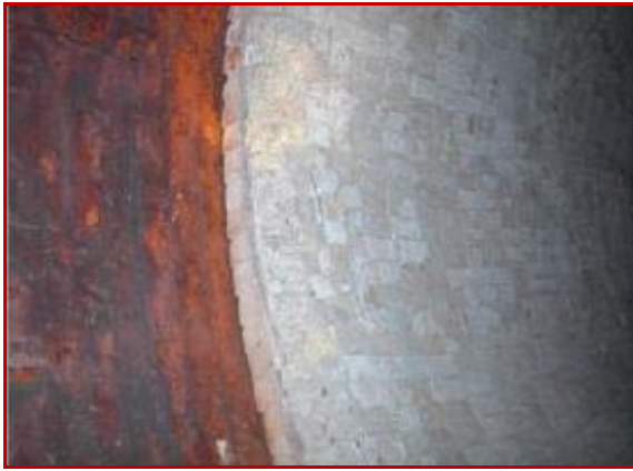
Figure-37: Corroded high temp area of kiln shell after removal of brick lining
